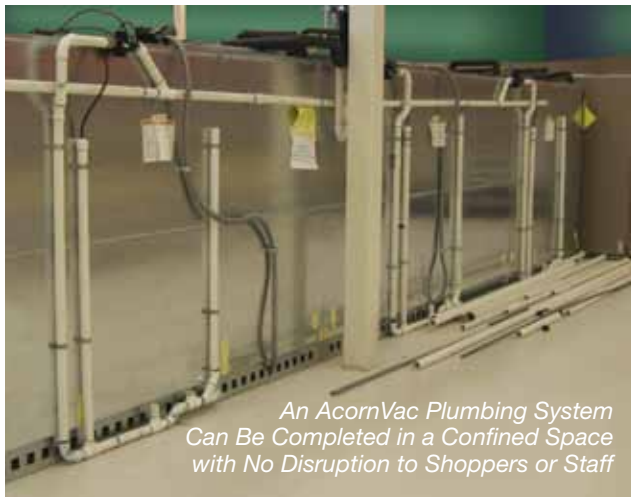
Back view of a vacuum plumbing system installation on a refrigerated case
