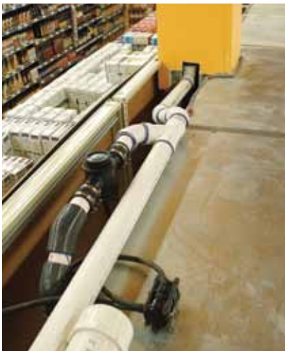
Top view of a vacuum plumbing system installation on a refrigerated case
